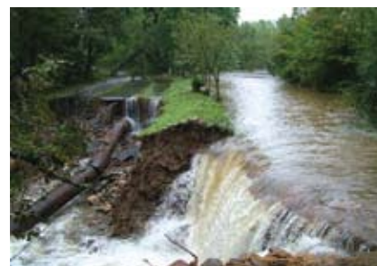
Damage to the city water system in Asheville, North Carolina, due to heavy rain in 2004.
