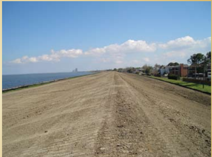
Recent upgrades that raised the height of this earthen levee increased protection against storm surge in the New Orleans area.
