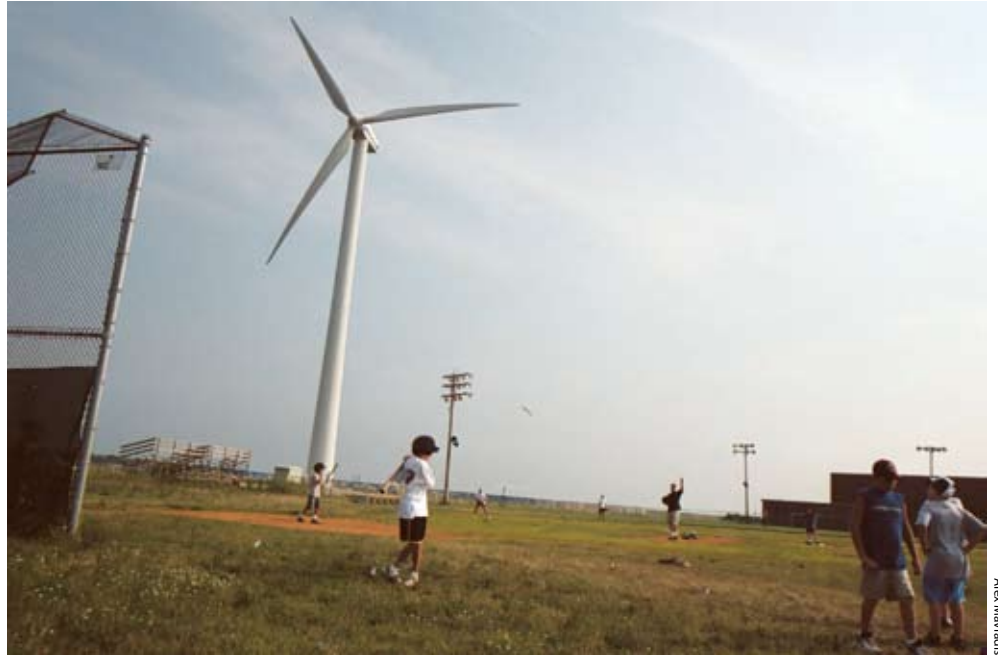
This 600-kilowatt wind turbine went online in Hull, MA, in December 2001. Wind energy represents one of the most attractive near-term options among renewable resources for making substantial, relatively low-cost contributions to electricity generation in the Northeast.
